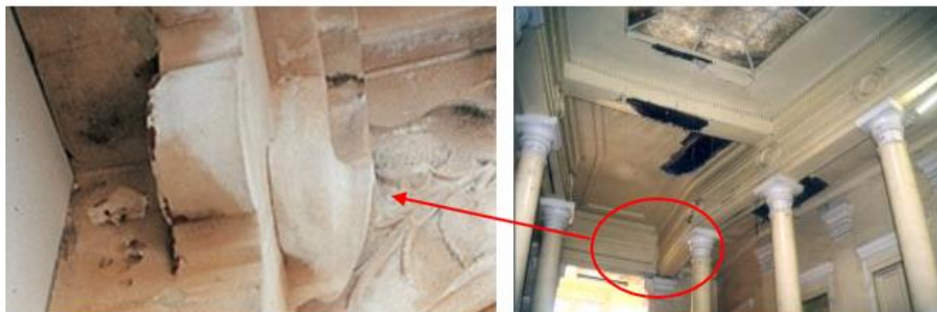
Fig. 6. Efflorescence on the Main Entrance
