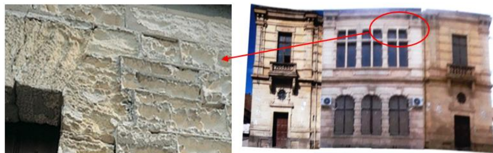
Fig. 5. Dissolution on the South East façade
