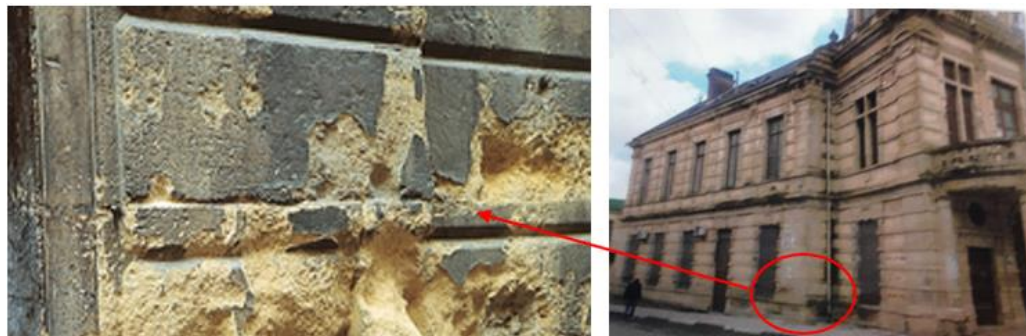
Fig. 4. Alveolization on the North Facade
