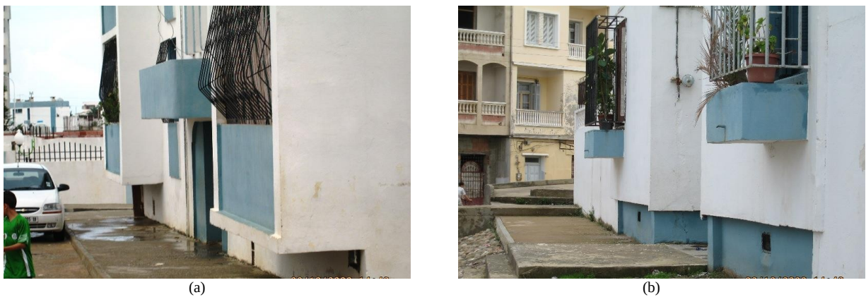
Figure 11. Extended balconies obstructing pedestrian circulation on the sidewalk (a). Concrete flower boxes positioned at very low heights (b), causing inconvenience and sometimes leading to accidents in « Camp Chevalier » district (Jijel city).
