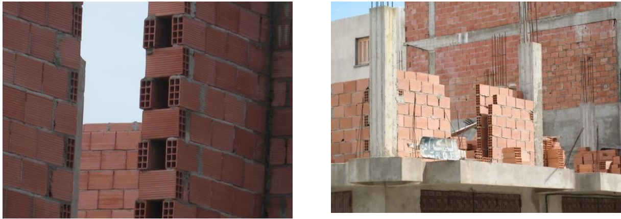
Figure 8. A poorly executed cavity wall in the Herraten district, in the suburbs of Jijel, constructed for cost-saving reasons but at the expense of thermal comfort and overall building performance.
