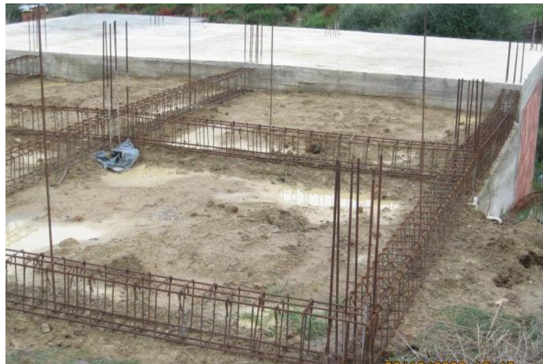
Figure 12. Poor execution of a foundation in Herratene: the reinforcement bars of the ground beams are placed directly on the soil, without a blinding concrete layer.
