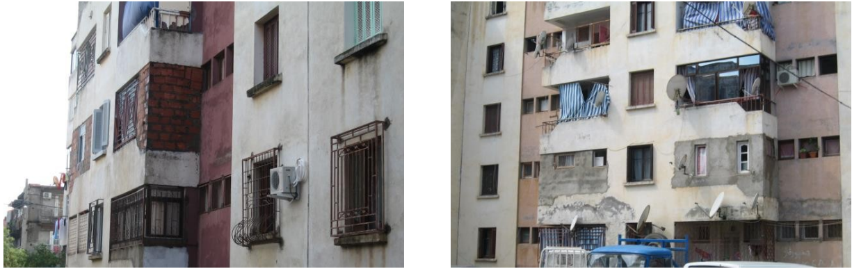
Figure 10. Spatial appropriations (modifications) of public building façades (balconies) without authorization in 400 housing district (Jijel city).
